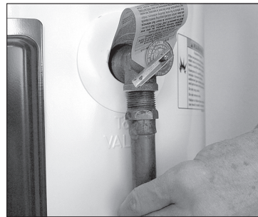
The T&P Relief Valve discharge pipe must be installed properly and piped to an adequate drain.
