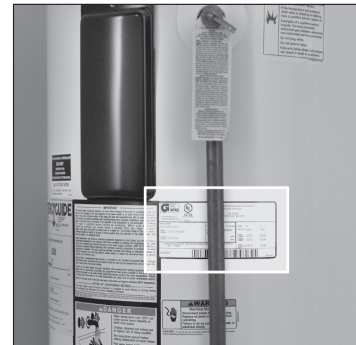
The water heater’s electrical requirements can be determined from the data plate.
